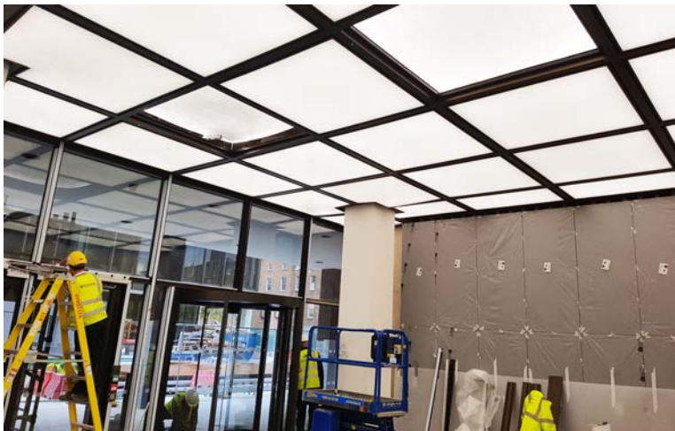
Installing the Custom LitePads into a rectilinear grid in the ceiling. Photo: Mark Reilly, Arup-Ireland
